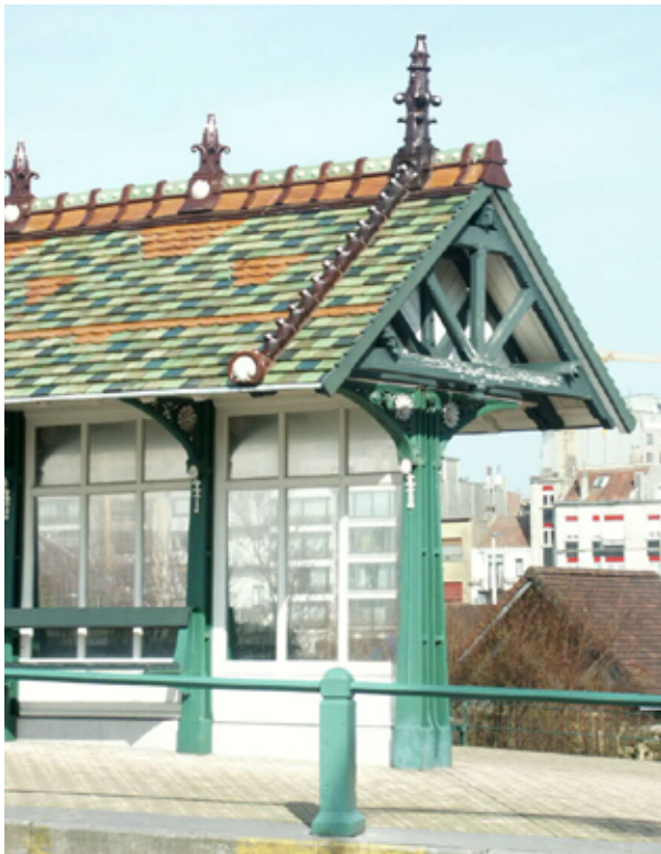
Example of roof tiles aged 115 years and still in use: Blankenberge shelter (part renovated in 1993) ( https://beeldbank.onroenderfgoed.be/images/25742 )
