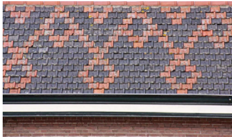
Concrete example of reuse of roofing products (natural slates): see https://opalis.eu/nl/inspiration/5599
