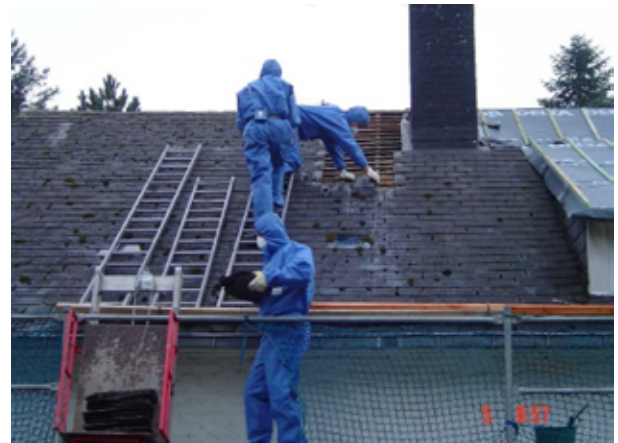
Example of removal, at foot of downspout, of material containing asbestos and coming from roofing containing asbestos (photo OVAM, 2018)
