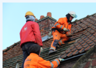
Example of submitting roof tiles to a "sound test" on removal (© Buildwise, Tuighuisstraat worksite, Courtrai)
