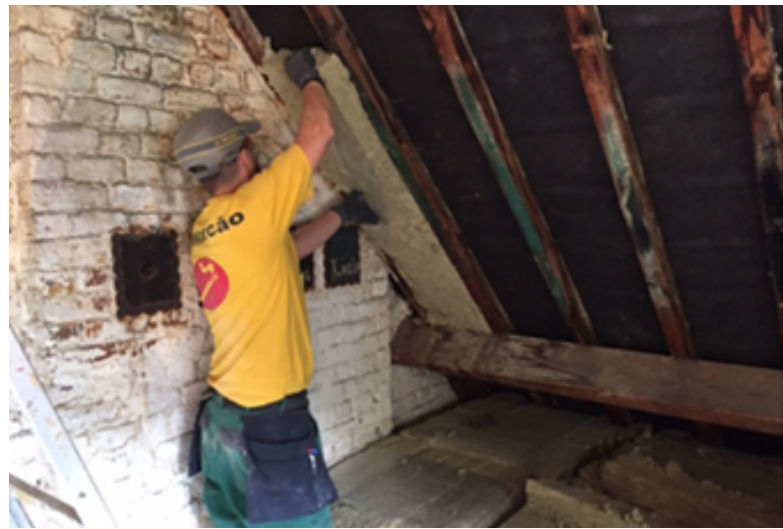
Reuse of mineral wool insulation from interior partitions of an office building in Brussels (ONSS)
