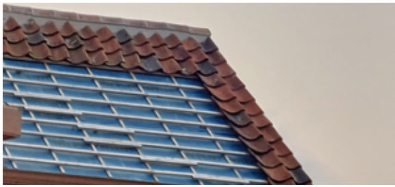
Example of traditional fixing (with mortar) of ridge tiles as part of a recent roof renovation (2023) while preserving the authentic appearance (photo F. Dobbels).
