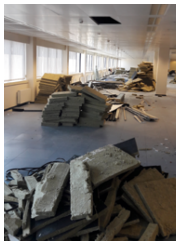
Sorting of mineral wool from internal separation partitions at the ONSS worksite in Brussels © Buildwise
