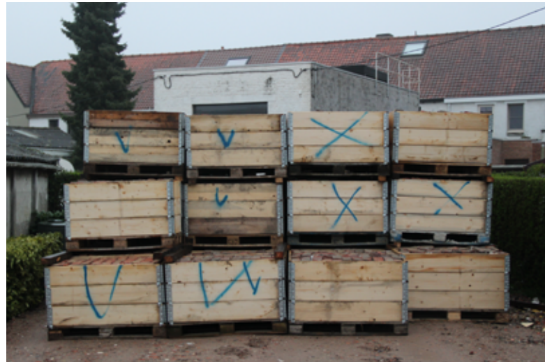
Bricks sorted on worksite into different bins according to compliance with required criteria –Tuighuisstraat worksite
