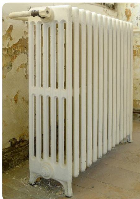
Column radiators - 'Classic' style
