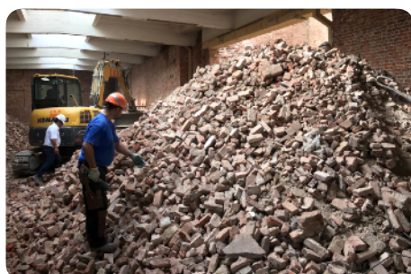
Demolition and reclamation on site. Renovation of the Tour A Plomb, Brussels. © BVDA - Bernard Van Damme Architecte
