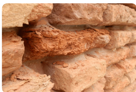
Crumbling brick, unsuitable for reclamation
